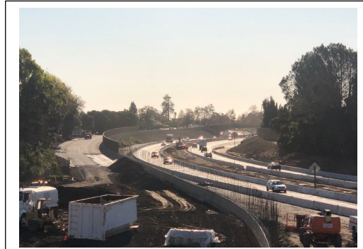
U.S. 101 is being widened to accommodate two extra lanes throughout the City's extent, with improvements proposed for each interchange with local streets.
