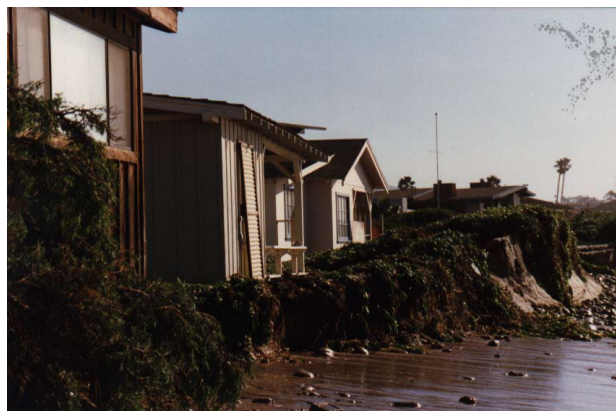
The 1983 El Niño event resulted in major damage to beachfront homes along Carpinteria City Beach, near Ash Avenue. Without adaptation, future storms in combination with sea level rise could result in severe erosion of the beach and repeated damage to shoreline structures.
