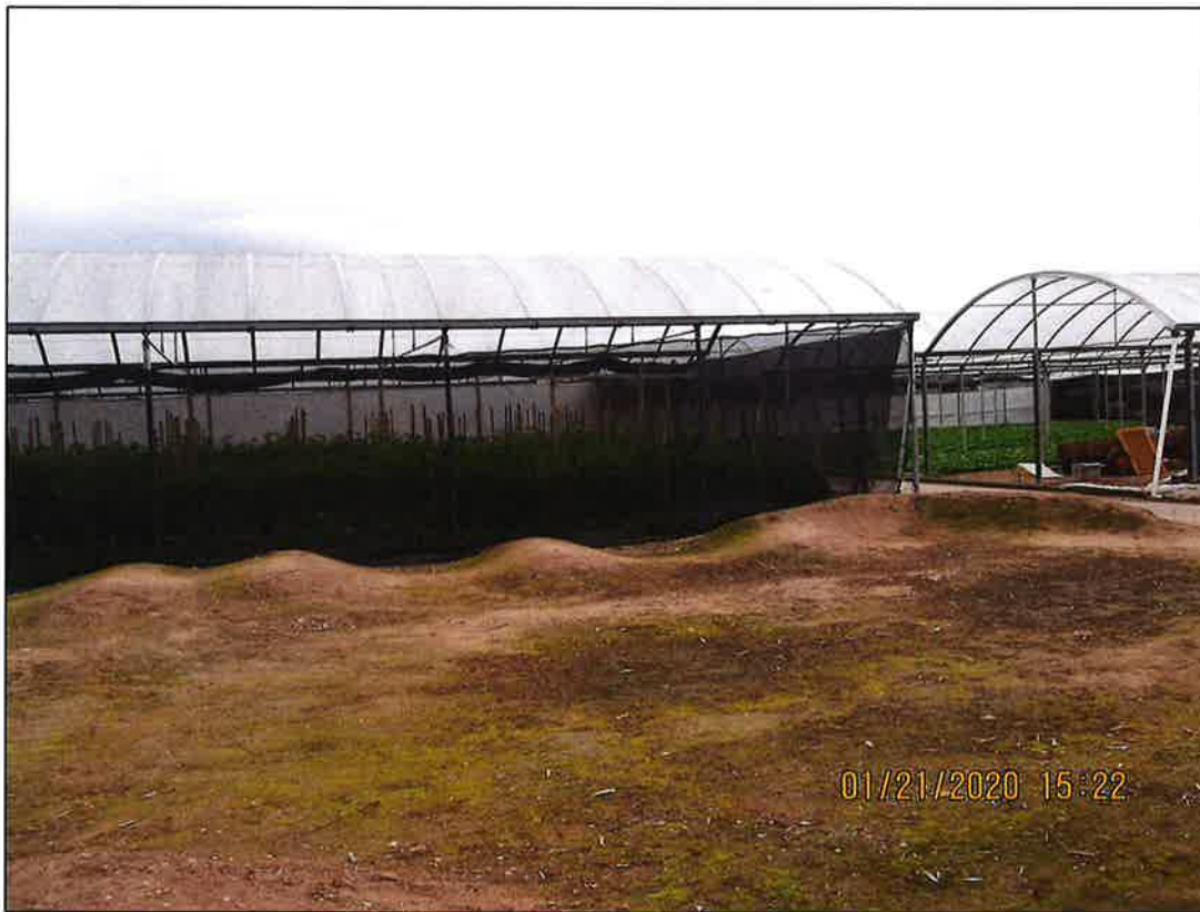
The above greenhouses, located at 1552 Casitas Pass Rd (APN 001-060-040) have a pending permit (19CDP-00000-00058) to utilize these open-sided "mixed light" structures for cultivation of cannabis.
